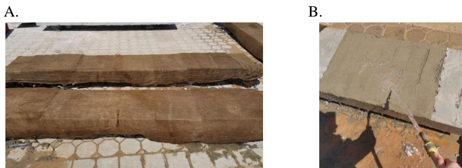
Figure 3.19: Curing of of FRCM composites: A. Beams covered with burlaps, B. Spraying water on the burlaps
