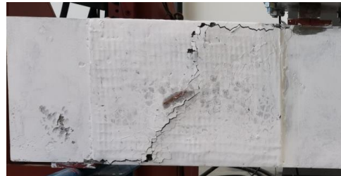
Figure 4.14: Crack pattern of specimen ST-G1-90: A. Picture of the beam at failure, B. Close views of the crack pattern (west shear span)
