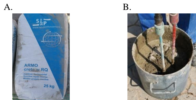
Figure 3.17: Preparation of the cementitious mortar: A. Solid cementitious material, B. Mixing of mortar
