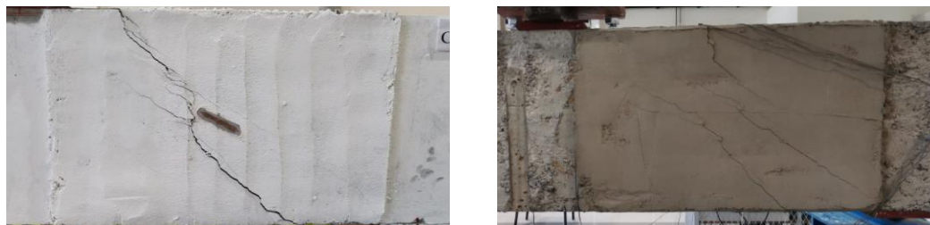
Figure 4.10: Crack pattern of specimen ST-C1-90: A. Schematic drawing of the crack pattern, B. Picture of the beam at failure, C. Close view of the crack pattern (east shear span)
