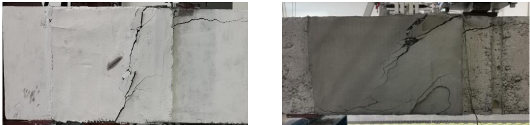
Figure 4.8: Crack pattern of specimen NS-C2-90: A. Schematic drawing of the crack pattern, B. Picture of the beam at failure, C. Close view of the crack pattern (west shear span)
