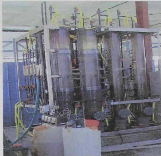
Figure 4-10: Dual media filters (Ondeo pilot plant)
