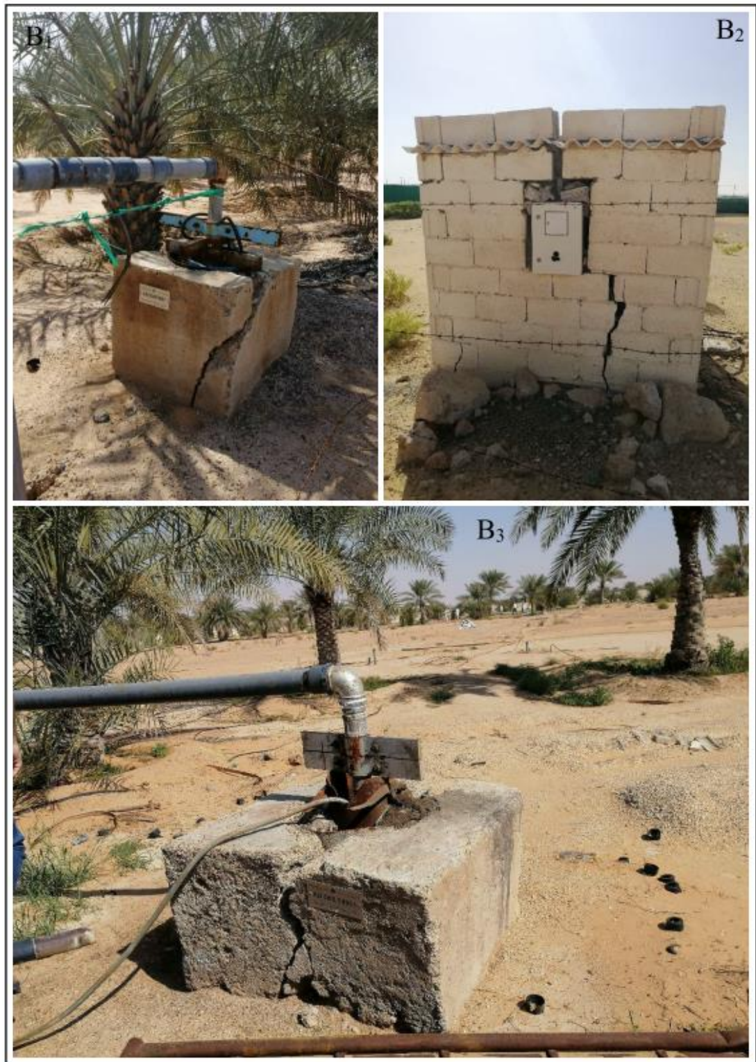
Figure 4.5: Examples of constructions protrusion due to land surface subsidence.
