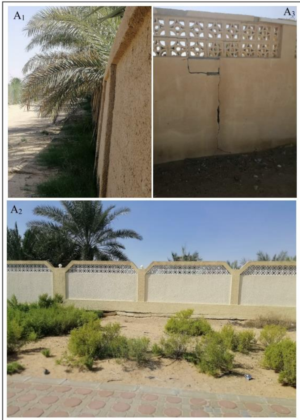
Figure 4.4: Examples of differential settlements of the construction's foundations.
