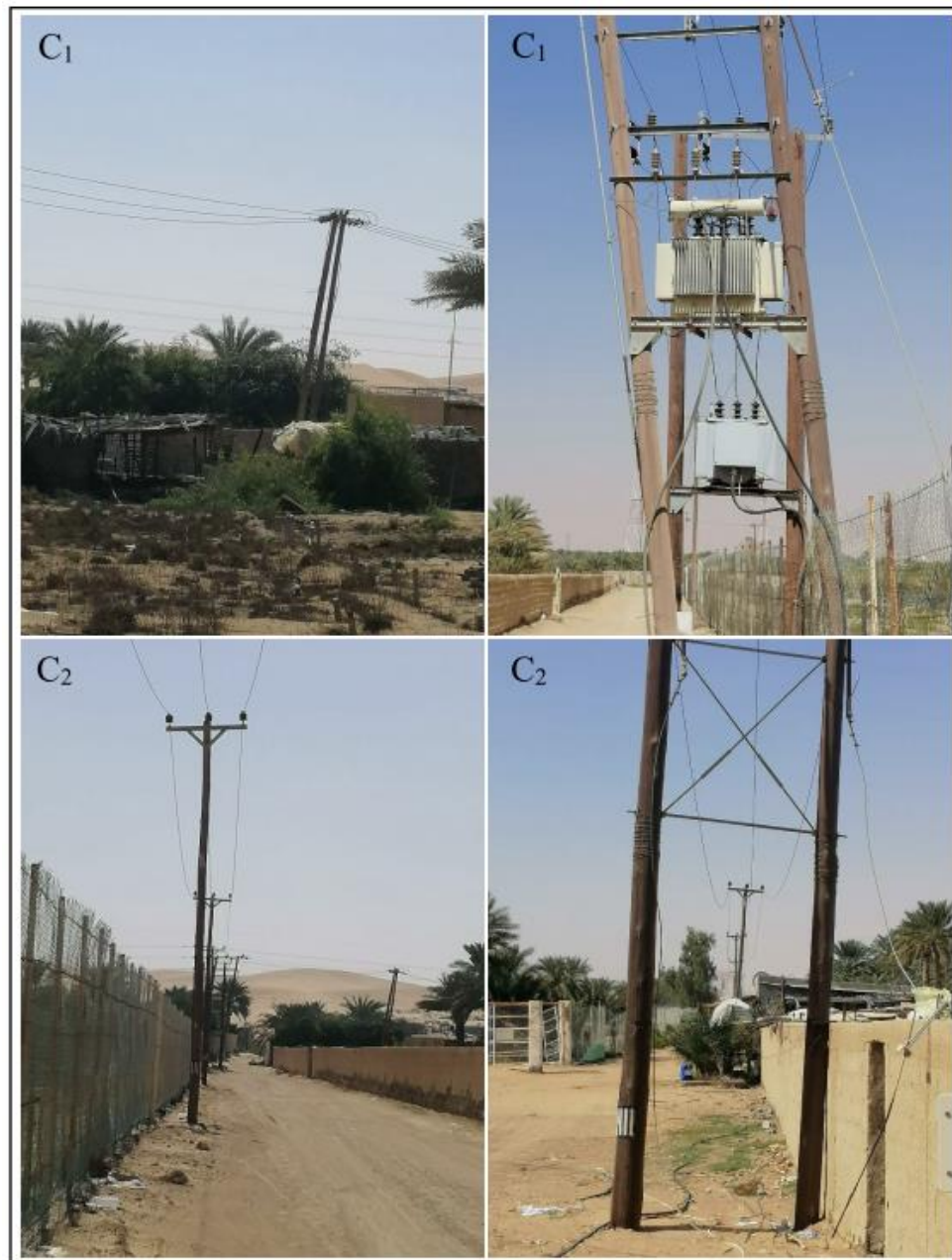
Figure 4.6: Examples of inclined electrical pillars.
